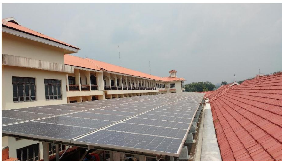
Photographs of 50 kW solar power plant installed on roof top
